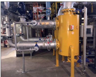
Figure 1. Closed steam-water heat transfer stations
