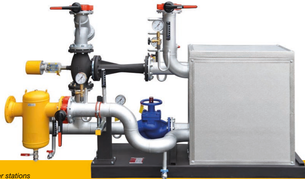
One of the heat transfer stations with plate heat exchanger and jet pump
